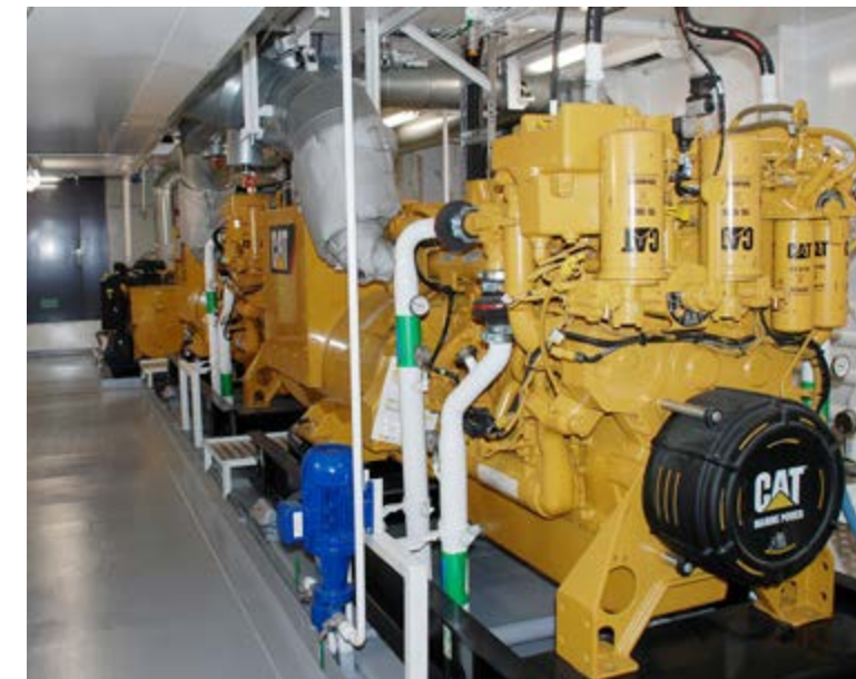
Auxiliary power room.
