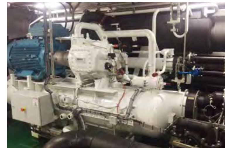
New ammonia RSW system.
